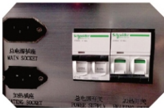
seperate machine heating power supply
