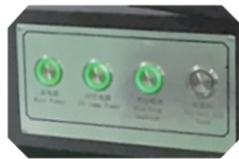
Automation Integrated Control Panel
